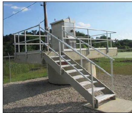
Photo 16. Elevated lift station, with proper safety railings and security fence (Source: Excel Fluid Group)
