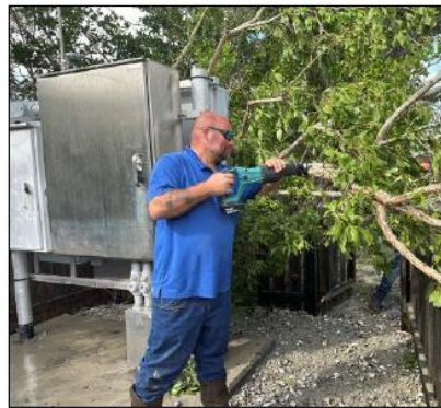
Photo 15. Public Utilities removing debris after Hurricane Helene
