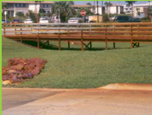
Dry retention pond
