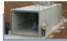
STORAGE CONCRETE CHAMBERS
