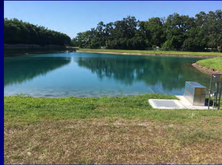
Water recirculation pump
