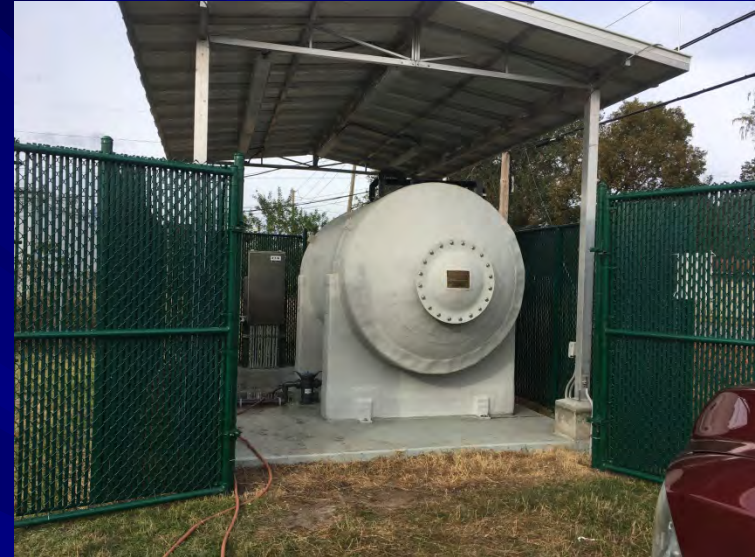
1,500 gallon Alum Storage Tank
