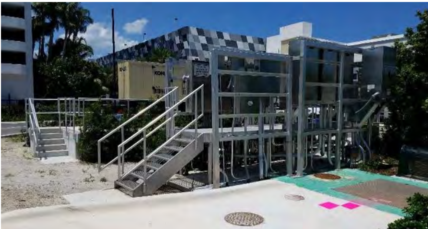
Elevated roads and pump station
