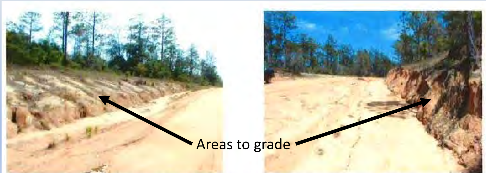
Figure 2-1. Severely Eroded Unstable Roadside Slopes (Photos by Mike Rainer)
