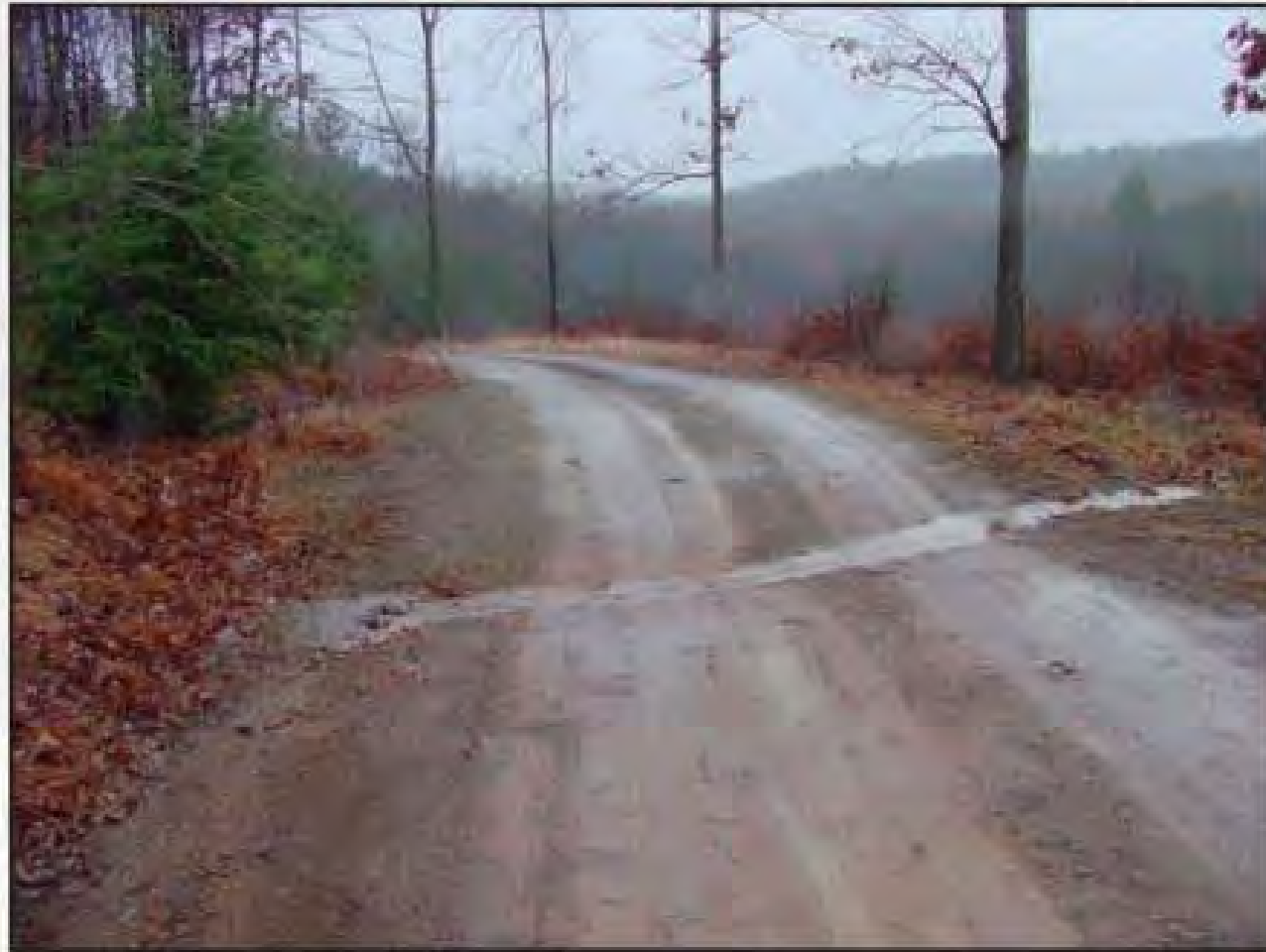
Figure 3.10—The broad-based dip pictured here conveys water from the road surface and upslope ditch into a vegetative filter area on the right.
