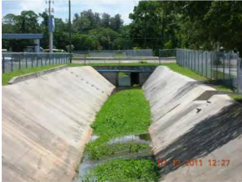
Figure 6: Ditch #5 in Pinellas County, Florida, is a manmade stormwater conveyance that discharges through a wetland into a navigable creek. It is already regulated as a point source. Under the Rule, it will be additionally regulated as a “water of the United States.” Fla. Stormwater Ass’n Comments 13
