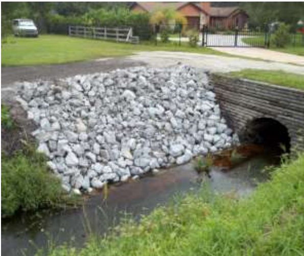
Tomoka Farms Roadside Ditch
