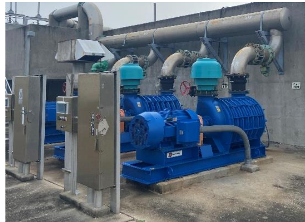
Blowers, Motors and Control Panels
