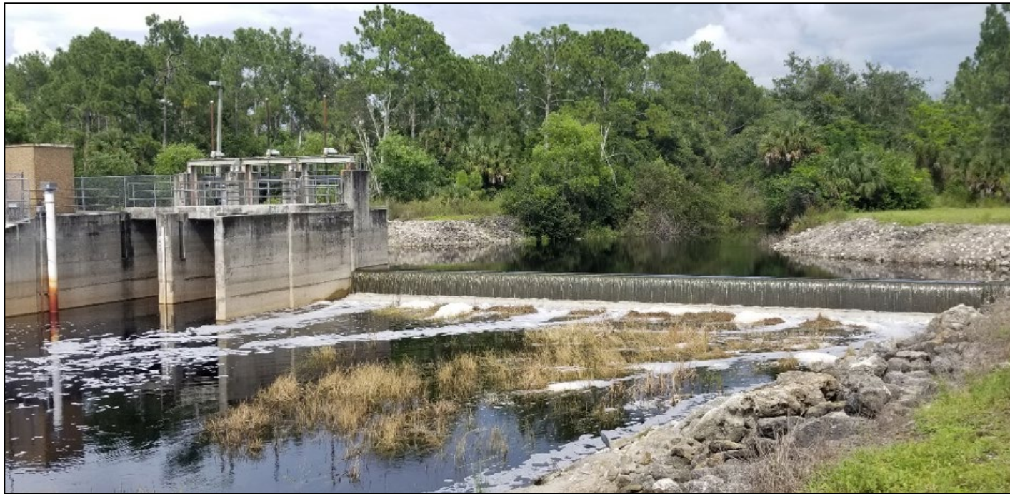
Kehl Canal Structure – 80-foot fixed crest weir and (3) low flow gated weirs
